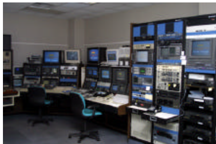
AT&T IVBN master control
